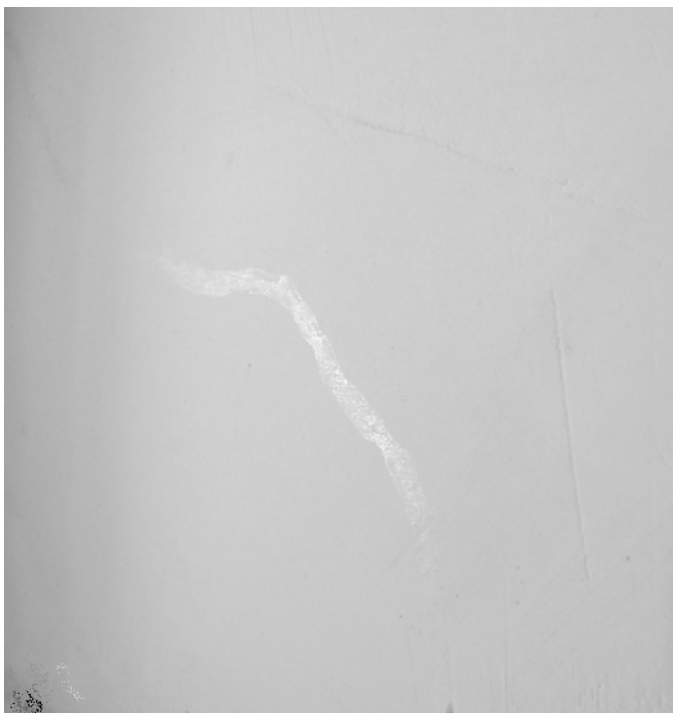
Figure 6. Mucus track on a wall in the basement of the National Research Restoration Centre of the Ukraine.
